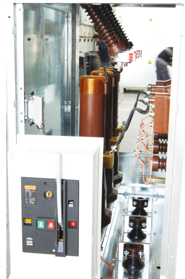
Cable Compartment of Cubicle with Circuit Breaker
