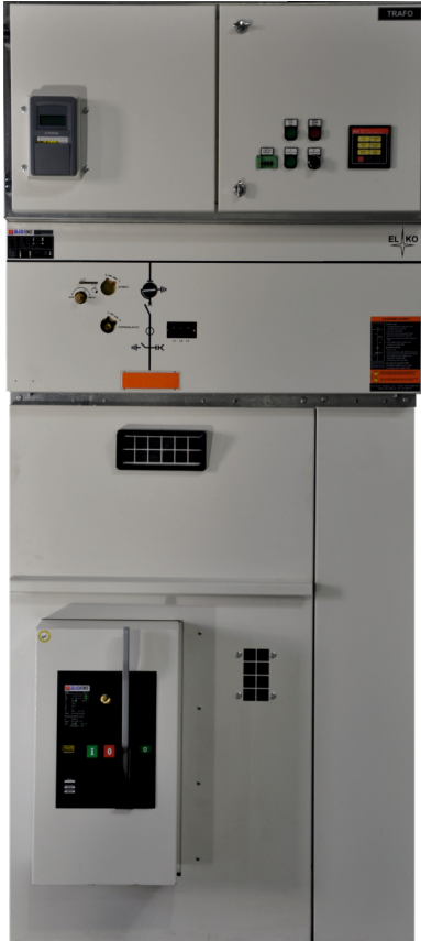
Cubicle with circuit breaker
